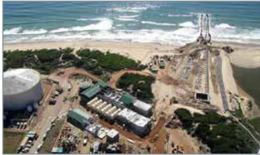
South Africa's largest desalination project - 15 MI/day Mossel Bay plant, under construction in 2010. Photo credit Royal HaskoningDHV.
